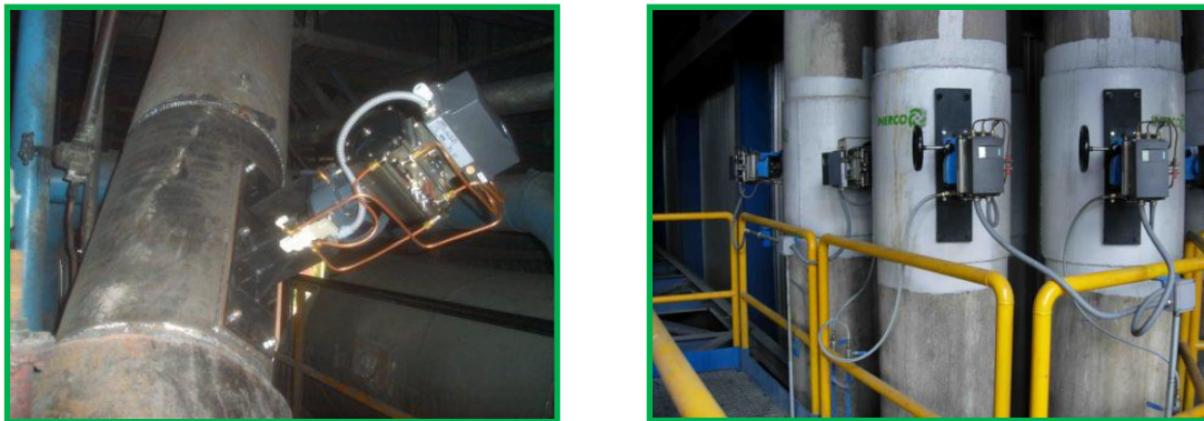
Figure 1: Automated ABACO-Coal dampers for coal flow balancing supply
