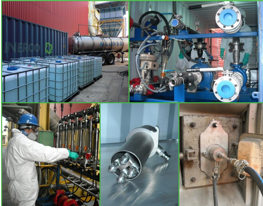
Figure 6: Images of the Advanced SNCR demonstration plant
