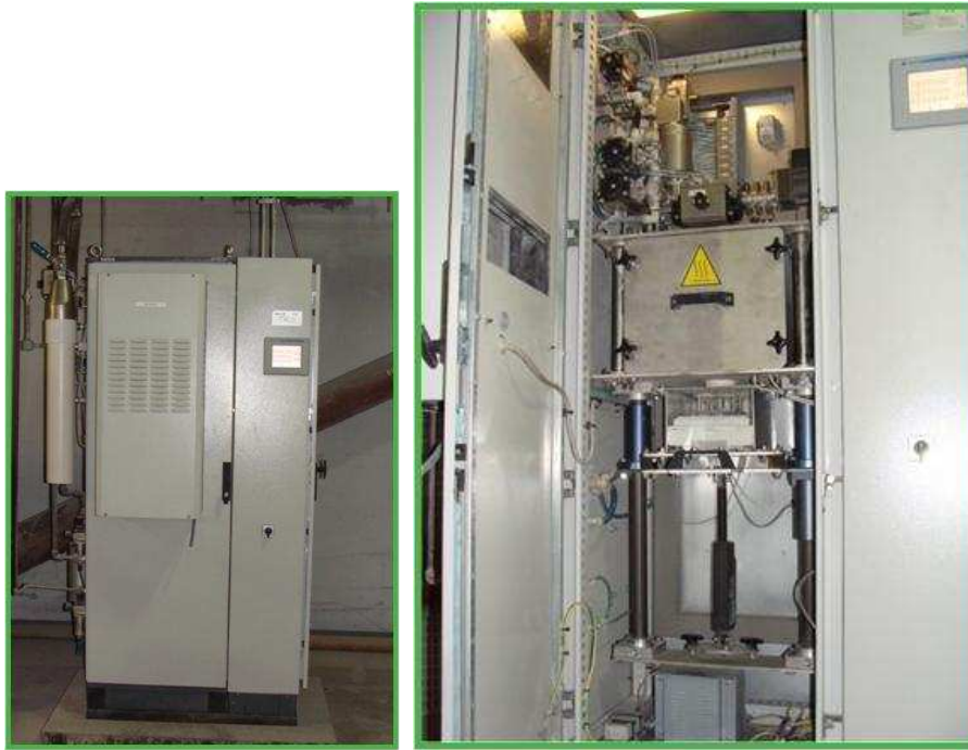
Figure 3: LOI Monitor for the online unburnt carbon-in-ash measurement
