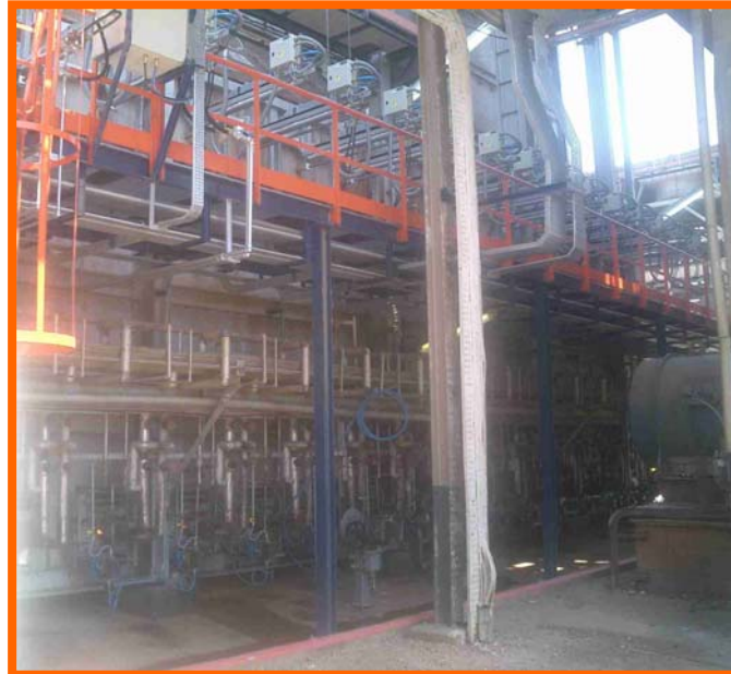
Figure 5: Particular arrangement of ABACO for CH1-B furnace of CEPSA-La Rábida Refinery
